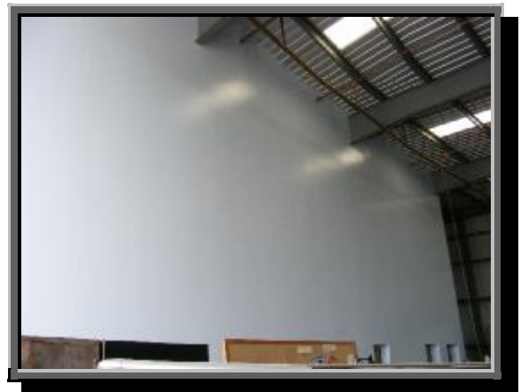
Here's the completed wall with the first coat of paint. Plans are in the works to have an aviation mural painted on the wall – with all our aircraft represented.
