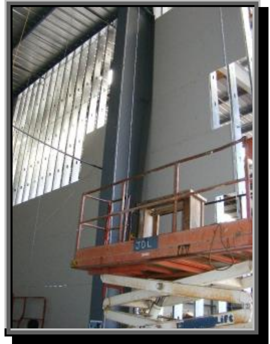
This shot, taken between the outside wall and the new wall, shows the existing girder and the dry-wall being installed.
