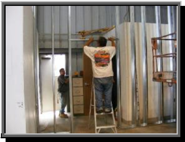
Workmen installing framing for one of the doors in the new firewall. The men's and women's rooms were left intact, with the framing forming a separate wall on the west side of them.
