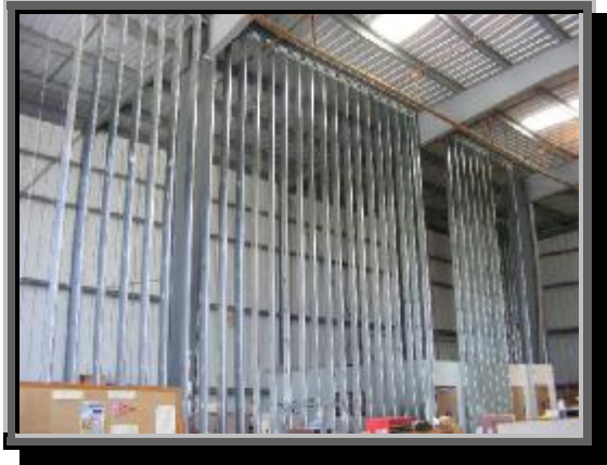
The metal framing partially up – all the way to the hangar ceiling.
