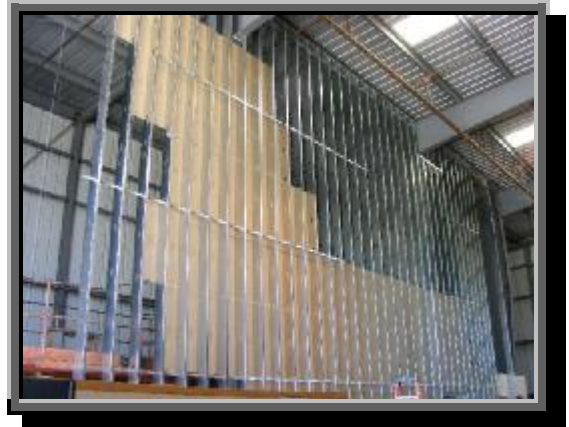
Insulation being installed before the dry-wall goes on the maintenance hangar side of the wall.
