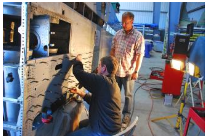
© Photo by Dan Newcomb Scott Drosos and Marc Russell attaching sheet metal to one of the PBJ's wings with clecos for later riveting.
