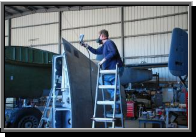
© Photo by Dan Newcomb Col. Mike Hohls applying paint to the PBJ's left wing. It is nearing the time when the wing will be attached.
