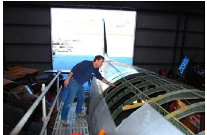
© Photo by Dan Newcomb Jeff Birdt working on removing the corroded "skin"
