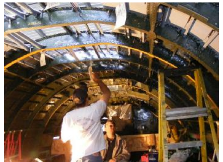
© Photo courtesy of Dan Newcomb Dan Newcomb and Scott Drosos riveting new panels.
