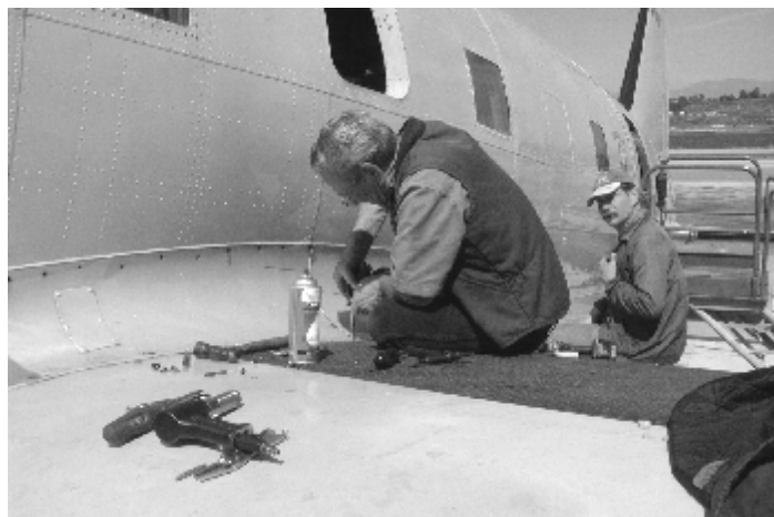
Laurence Allen (left) and Gary Koch remove fairings to gain access to China Doll's internal structure for NDI inspection
