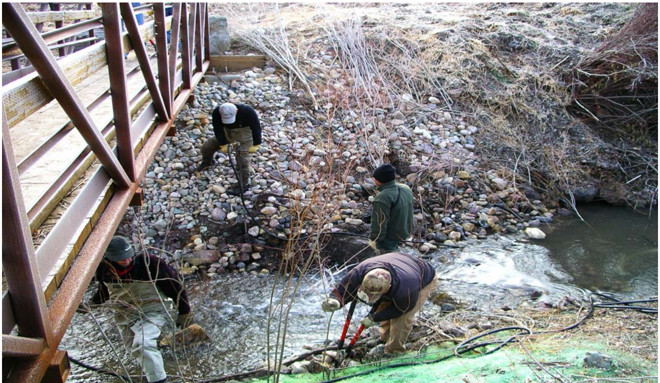
Water blasting was sometimes challenging trying to work the stingers down through the rocks. As the willows were placed into the holes, another crew came in behind and clipped back the willows to just a few inches.
